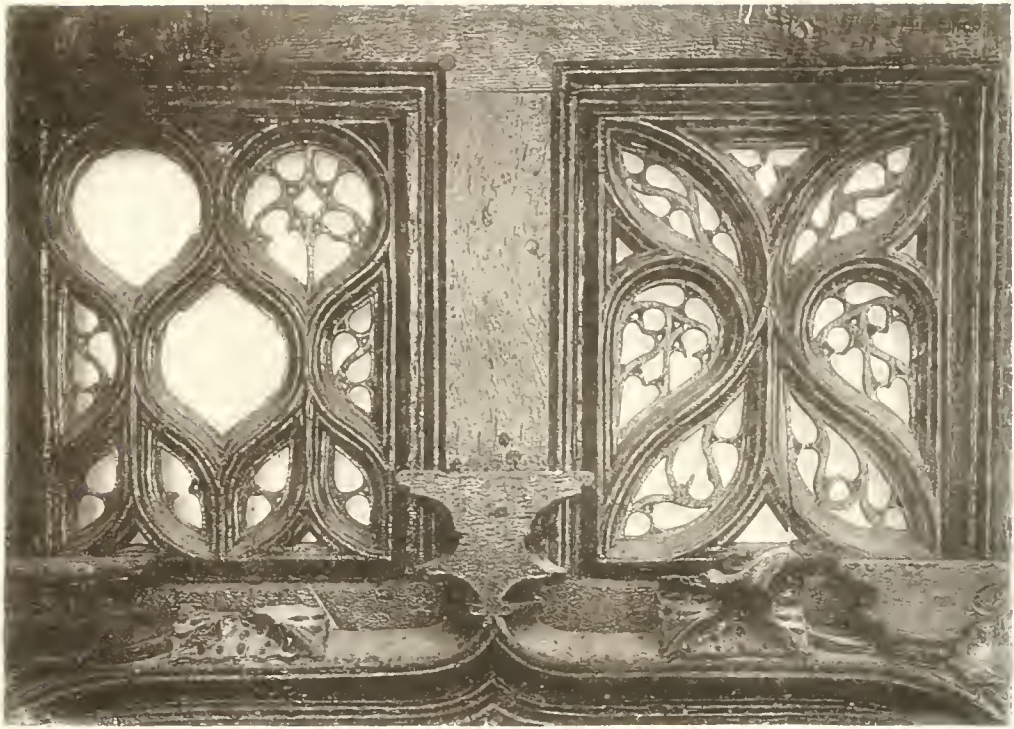
(A) FLAMBOYANT TRACERY PANELS AND PEDESTALS FOR ROOD AND FIGURES OVER DOOR BRUSHFORD SCREEN
